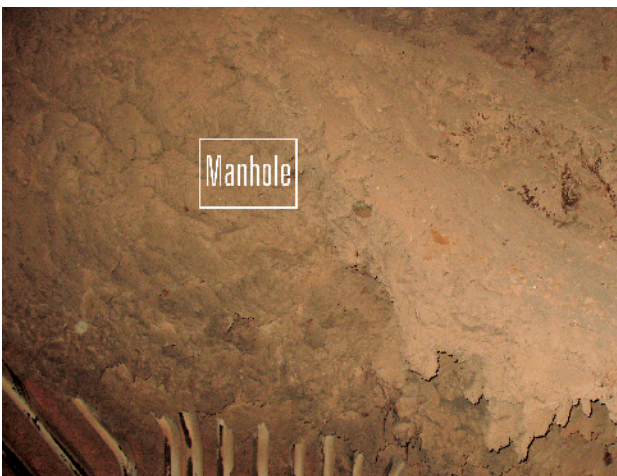
View of strongly fouled firebox after 5 days operation of untreated boiler.
